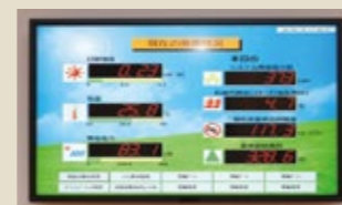
Solar power monitor
